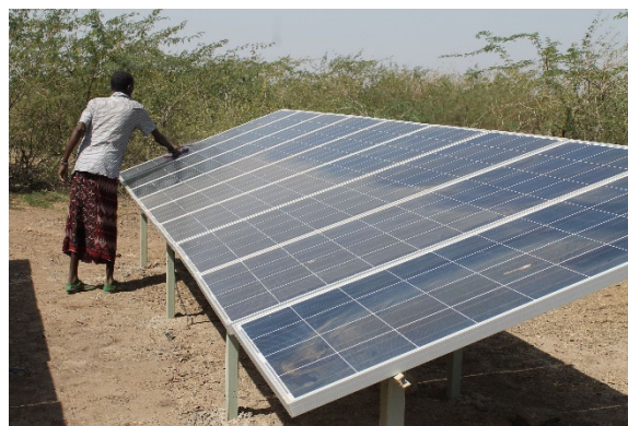
Operator cleaning solar panels at Be'eda water supply system in Gewane Woreda, Afar region. Photo Credit: Michael Tewolde.
