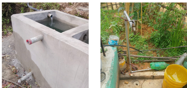
Sandhikharka one house one tap systems
